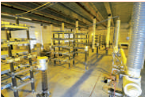
Interior of the Santa Ponsa converter station.
