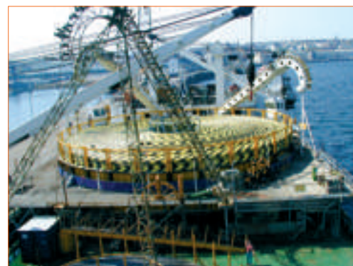
Submarine power transmission cable on the deck of the Giulio Verne .
