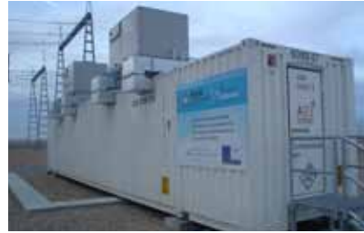
Lithium-ion battery installed in the Carmona transmission substation (Seville).
